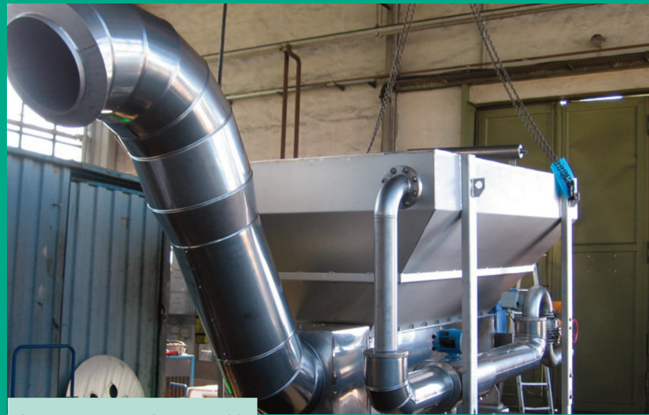
Septage Receiving Station FK100
