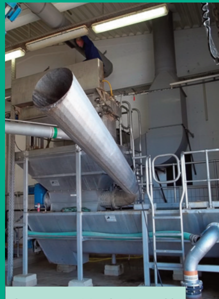
Septage Receiving Station FK100
